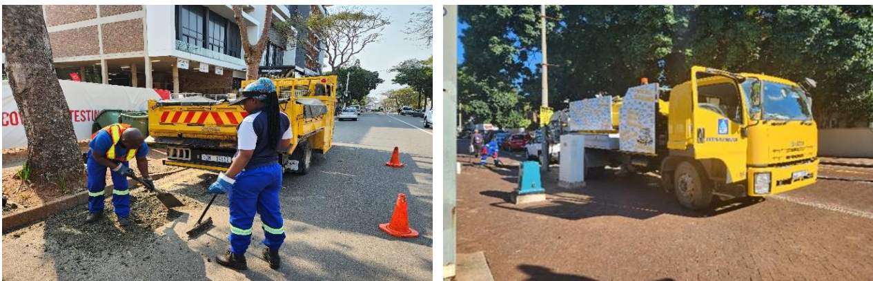
Photo above: Roads department backfilled and reinstated tar. Photo above: Roads and stormwater unblocked drainage point.
