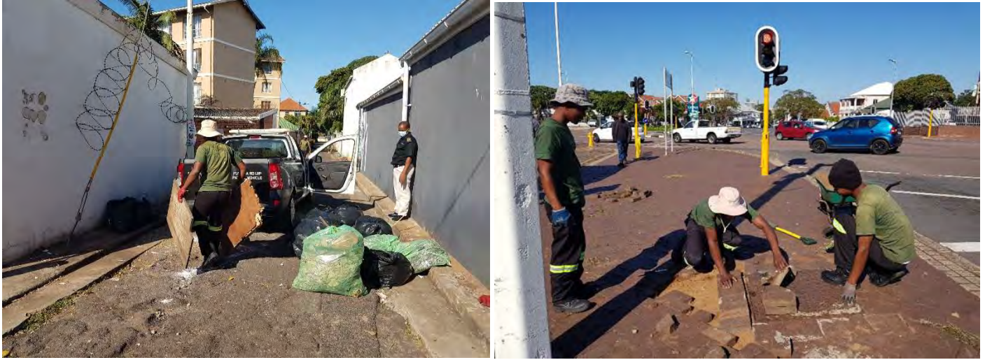
Photos below: Ongoing clearing and cleaning of service passages and repairs of damaged kerbs by cleaning team
